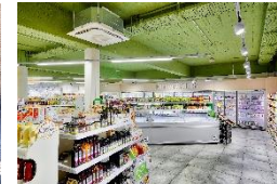
Retail Commercial refrigeration
