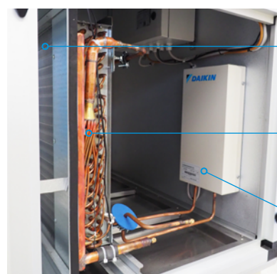
Return air grille with [M5] ePM10 55% filter
