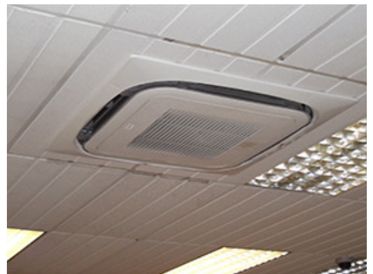
Picture above: Coral betting office self-cleaning cassette after 12 months use
